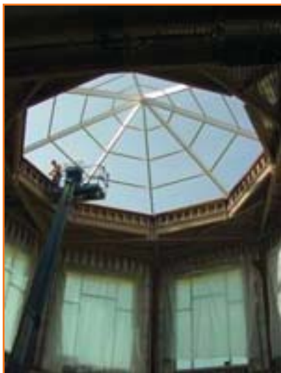
The new atrium skylight will be the focal point of Churchill Downs' new entry gate.
