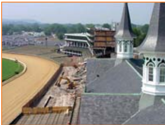
Phase II renovations in progress, as seen from atop the Twin Spires.
