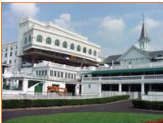
Phase I construction follows the grand historic style of the Twin Spires.
